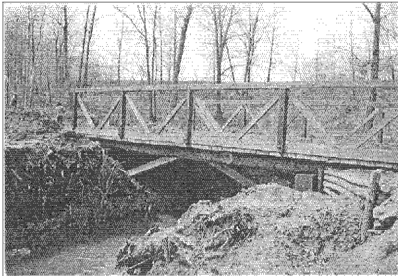
Figure 27: National Arboretum, View of Completed Bridge Over Hickey Run Creek, c. 1934. Source: "Narrative Report Covering Fourth Enrollment Period - N.A. Camp #1, Washington, D.C.," (3 April 1935), RG 79, NARA.
