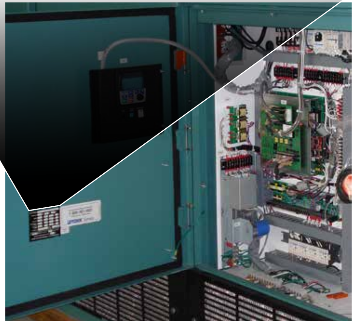
LOW VOLTAGE COMPARTMENT
