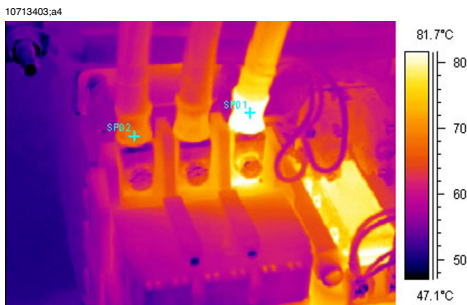
Figure 13.8 An infrared image of indoor electrical equipment (1)
