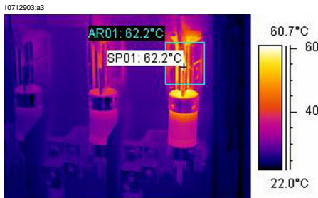
Figure 13.3 An infrared image of a fusebox where the maximum temperature is displayed
