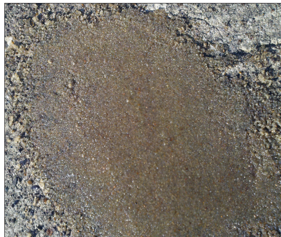
Pit patched with epoxy and sand
