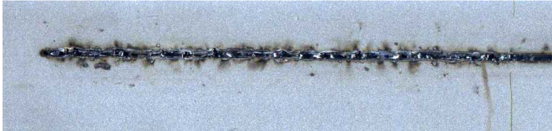
Figure 475: Splatter on surface caused by Zinc coating vapour blowout – Zero Gap between the welded panels 238
