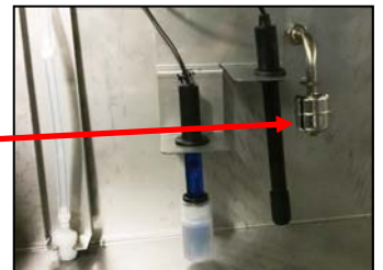
Fig. 2 Float switch/sensor; left side of reservoir; shuts off water once filled to proper level
