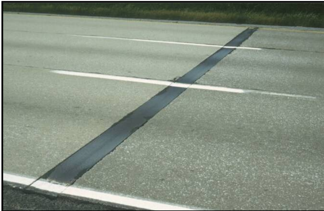
Good Terminal Joint – Do Not Count as Damaged
