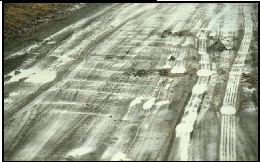
Corrugations – Medium Severity
