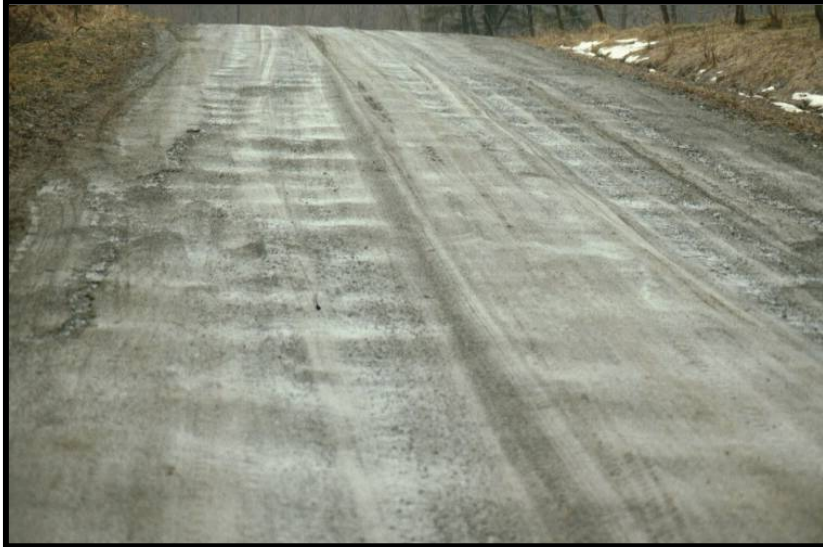
Corrugations - Low Severity
