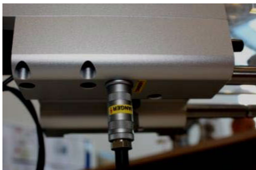
Figure 80. High-voltage cable connected to the ion source
