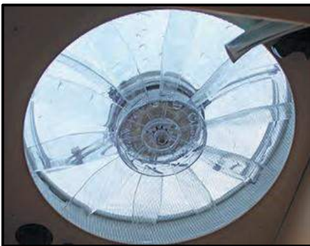
Figure 14-5: Overhead Vent Fan
