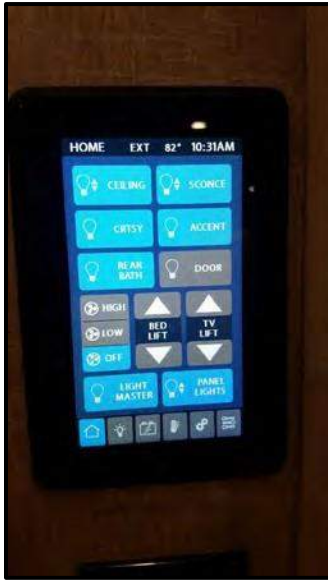
Figure 3-1: Spyder Controls Multiplex System
