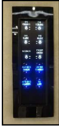
Figure 6-6: Television Lift Control Panel (located in the living room slide-out box)
