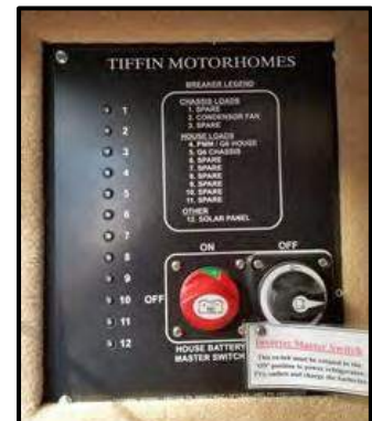
Figure 9-4: House Battery Disconnect Panel Switch
