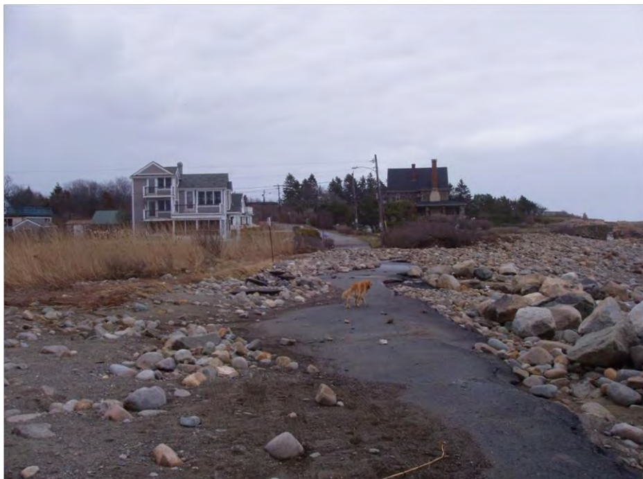
Photograph 4.5. Damaged pavement and overwashed sediment after a recent storm on a barrier beach. Photograph courtesy of Eric Hutchins, National Marine Fisheries Service.
