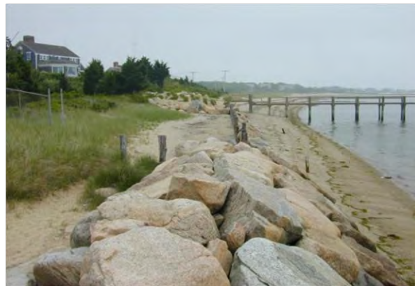
Photograph 1.9. Coastal dune with coastal engineering structures. Foreground: coastal dune landward of rock revetment. Background: coastal dune and beach landward of a deteriorated bulkhead.
