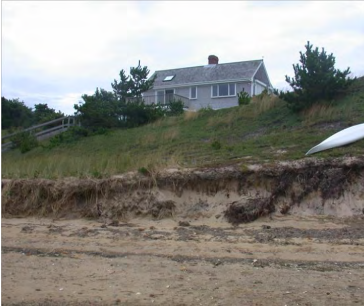
Photograph 1.12. Eroded scarp. The photograph also shows windblown-sand deposition in front of the scarp—a natural process of recovery after a storm. The only way to tell whether this is an eroded dune or bank is to look at the subsurface sediments behind/under the veneer of windblown sand to determine if they were wind or wave deposits (dune) or were glacial deposits (bank).
