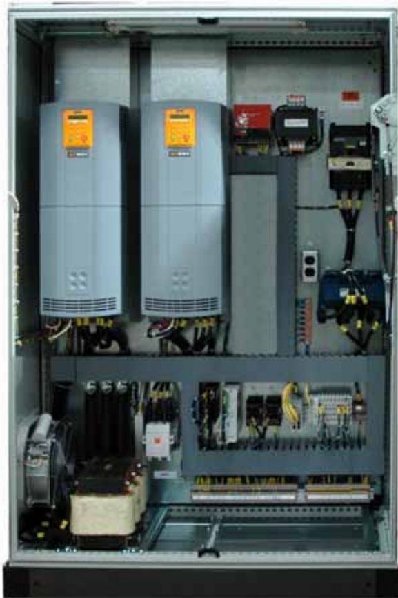
Illustration shows typical panel including AC690+ with AFE and additional system components.
