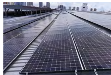
Photovoltaic power generation system at PA
