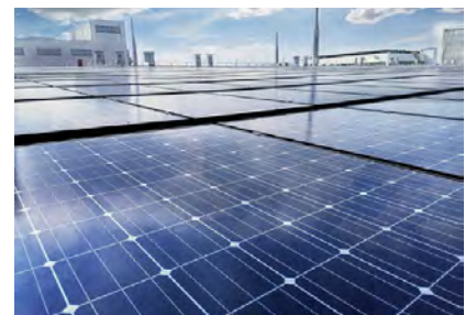
Photovoltaic power generation system at PIDMGZ
