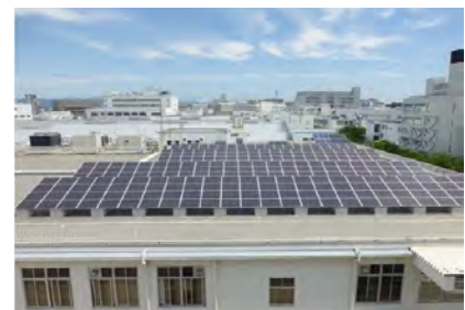
Photovoltaic power generation system at IS, Kadoma
