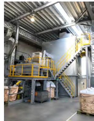
Compact crushing and sorting system for heat exchanger of air conditioner in PETECK
