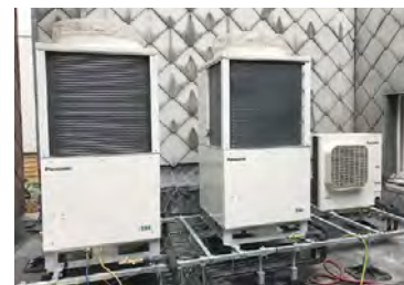
Example of two 10-horsepower freezer and one two-horsepower freezer at Carrefour Express (small stores)
