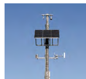
Coastal tsunami monitoring system in Higashi Matsushima City in Miyagi Prefecture
