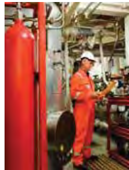
Fire safety equipment
