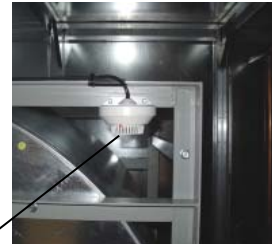
Smoke detecting probe
