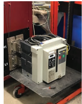
Primary Injection Testing
