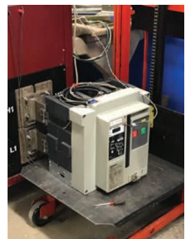
Primary Injection Testing
