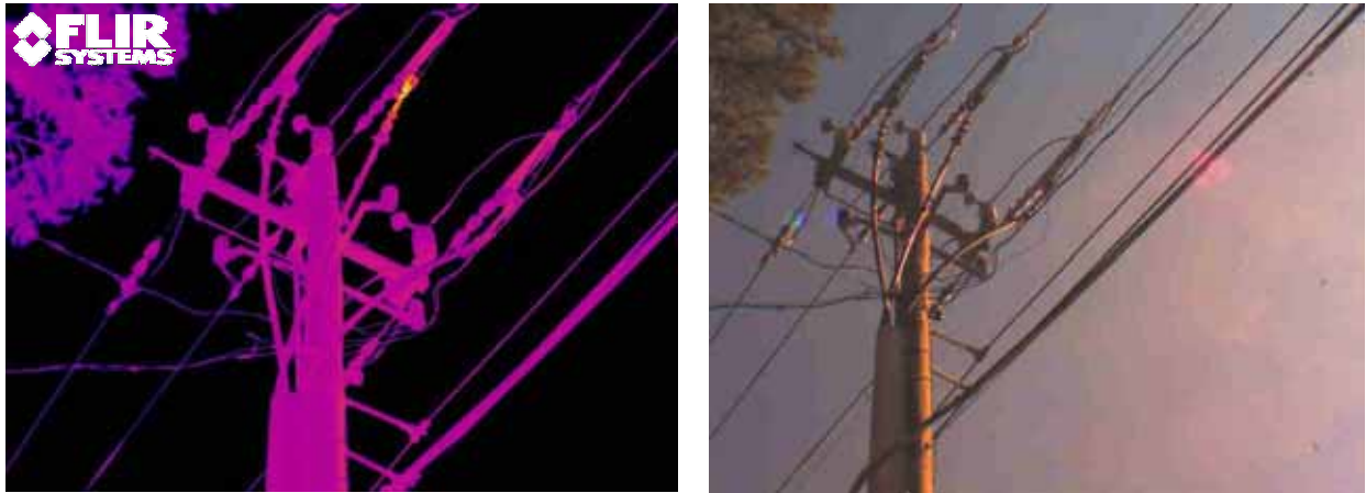
Figure 1. High resolution IR image and visual counterpart of a set of 23kV distribution switches. The center phase shows a significant temperature rise. Distance to target is 36 feet.
