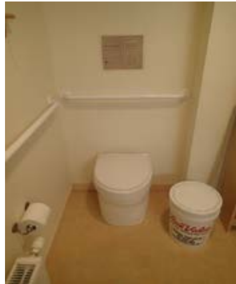
Composting Toilet, Shorey 2nd Floor, Spring 2013
