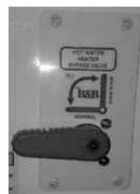
Water Heater Bypass
