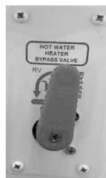
Water Heater Bypass
