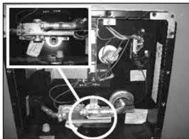
Fig 1: Water Heater Drain Plug
