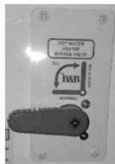
Water Heater Bypass
