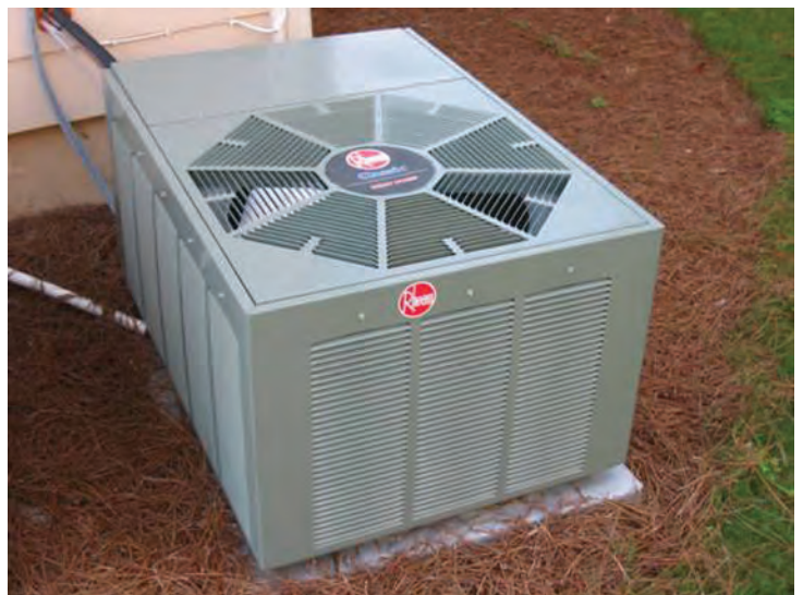
Figure 12.21. External Air-conditioning Condenser Unit
