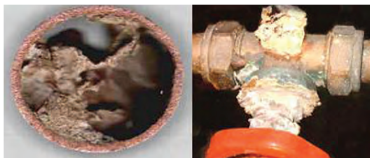
Figure 7.6. Corrosion in Piping Resulting From Galvanic Response
