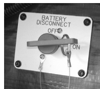
Battery Disconnect Switches
