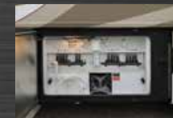
Berkshire's water manifold system with whole unit filter and exterior shower.
