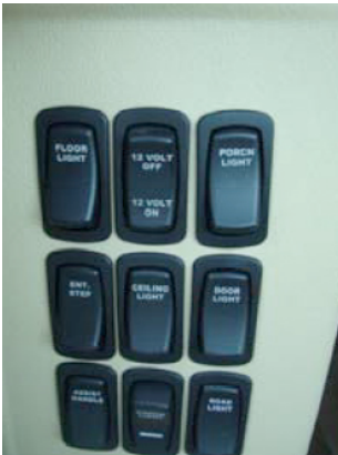
Figure 9-7. Entrance Step Switch (right middle)
