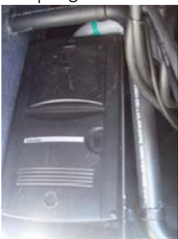
Figure 13-12. Vacuum Cleaner System
