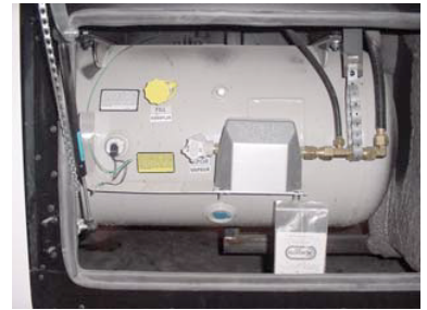
Figure 2-5. Liquid Propane Tank
