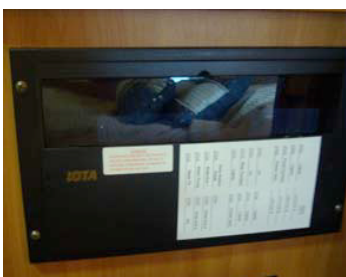
Figure 7-1. Circuit Breaker Box
