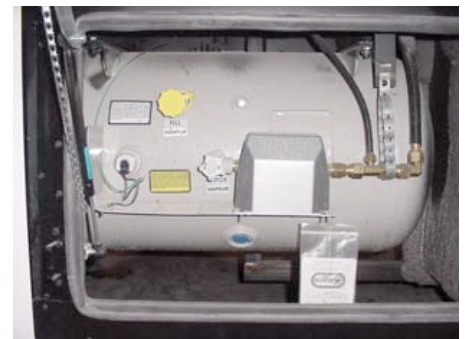
Figure 3-4. Liquid Propane Tank
