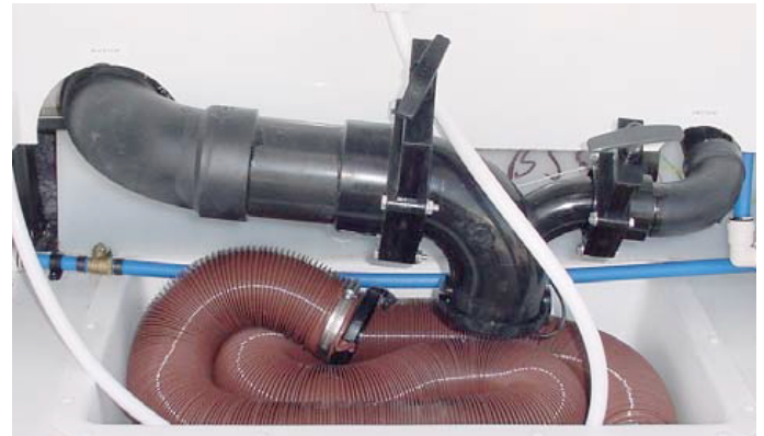
Figure 11-11. Sanitation Coupling, Valve, and Hose
