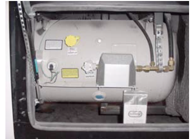
Figure 2-3. Liquid Propane Tank
