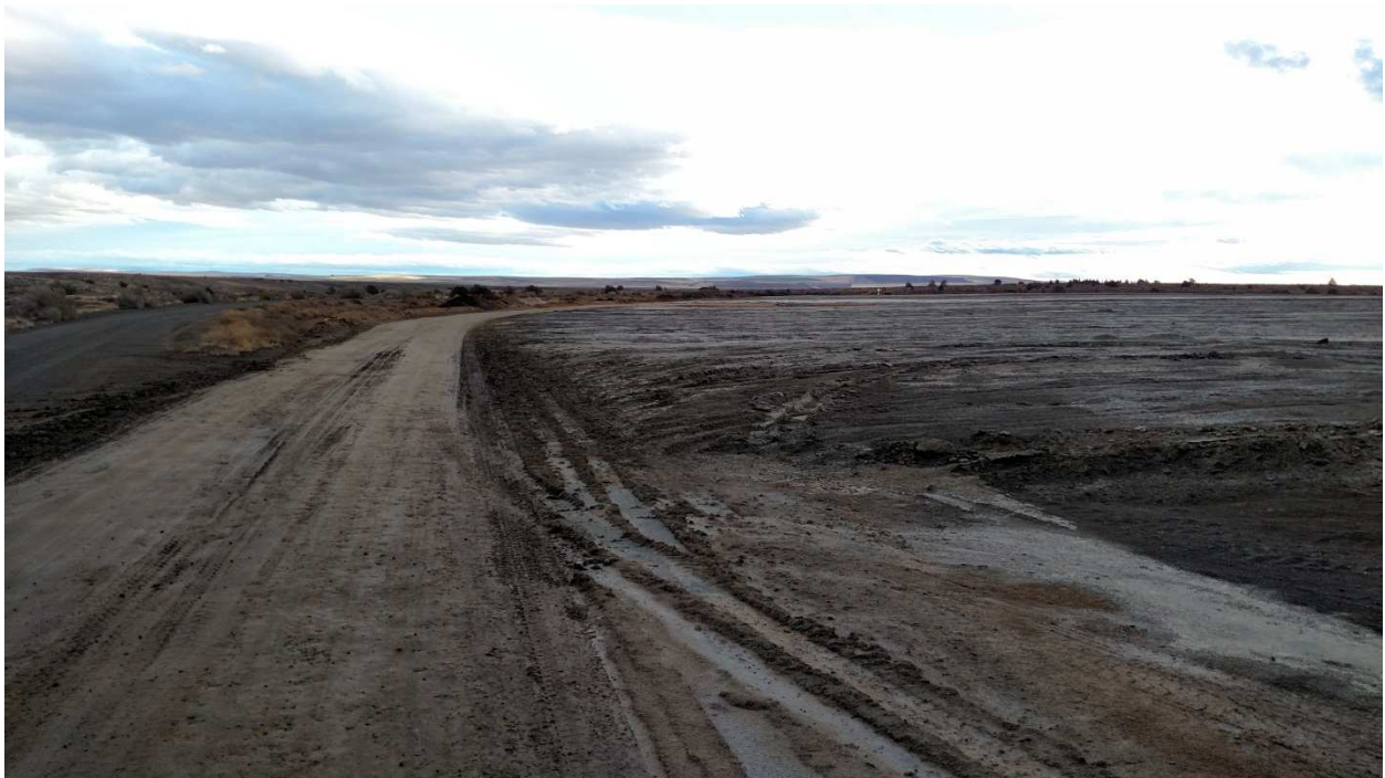
CCR landfill at northeast cornering, viewing south. Entrance to northeast side of landfill.
