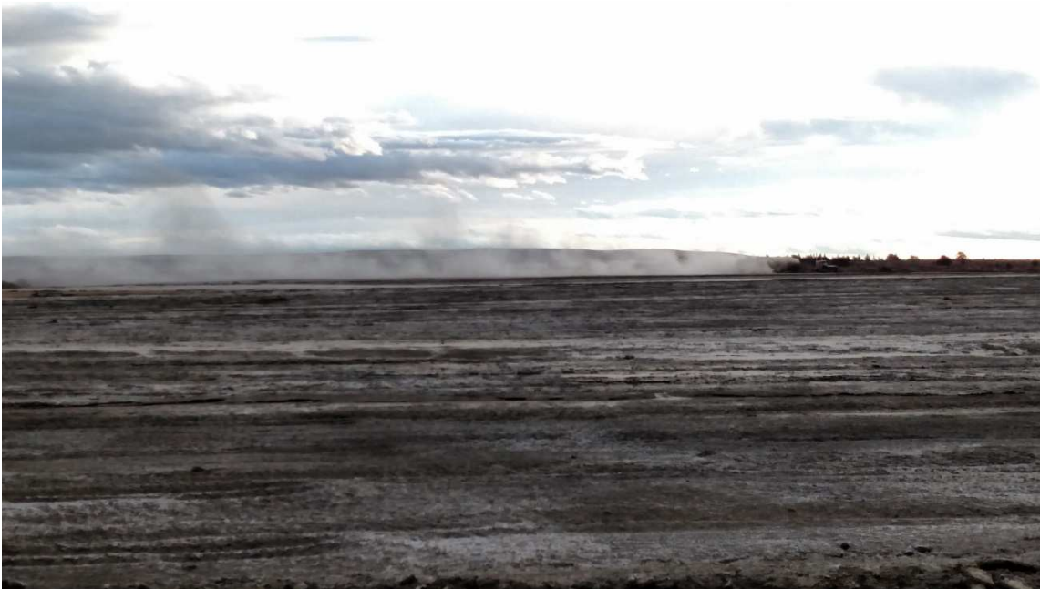
CCR landfill at north side, viewing south. Ash truck depositing fly or economizer ash.
