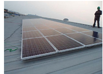
Photovoltaic power generation panels
