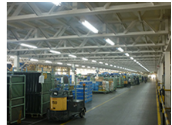
In-plant LED lighting
