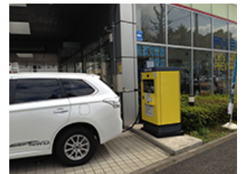
Quick charger installed in a dealer
