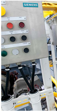
Figure 11-14 Conductors routed in raceways
