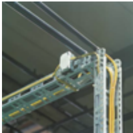
Figure 11-19 Example of exposed cables
