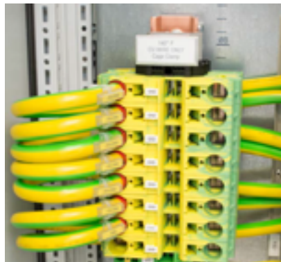
Figure 13-6 Siemens 8WH grounding terminals
