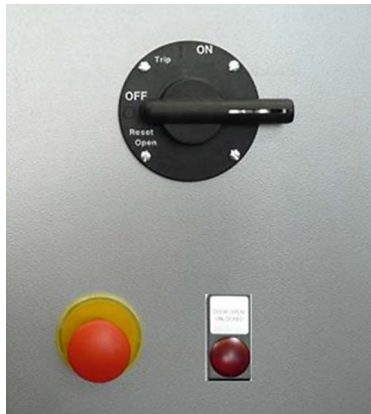
Figure 13-21 Front rotary operating mechanism for main disconnecting means
