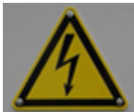
Figure 11-7 Example identification of an electrical enclosure
