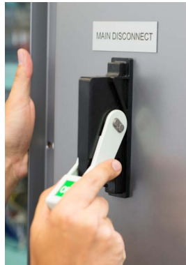
Figure 5-17 Example: Defeating without tools by actuating a lever on the reverse side of the door with the left hand.
