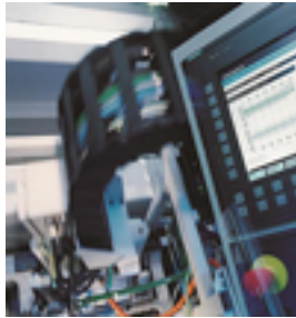
Figure 11-16 Drum cable example
