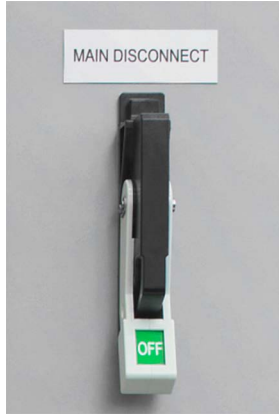
Figure 13-20 Toggle lever for main disconnecting means
