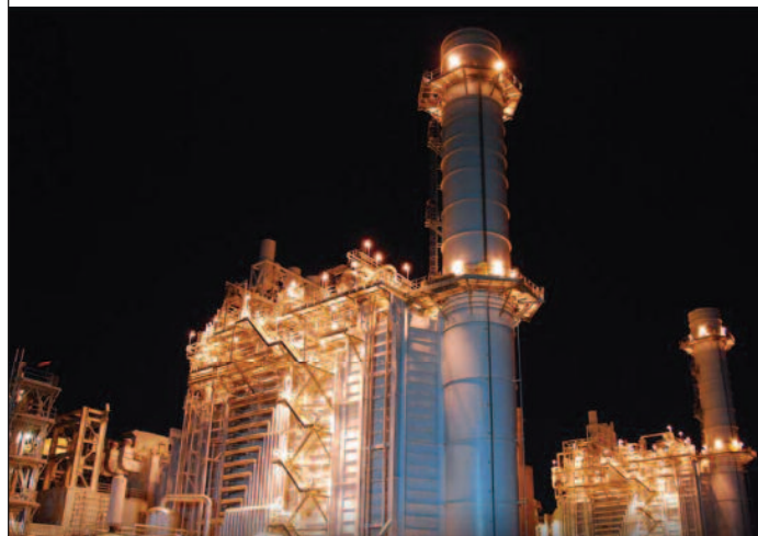
Figure 6. GE Engineers are available to visit sites and recommend exhaust upgrades.
