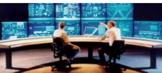
Control systems have many industrial and utility applications, including power plants, steel mills and pulp and paper factories.
