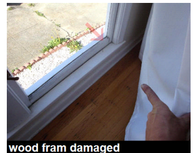
wood fram damaged
