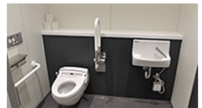
Toilet that can be easily used by people in wheelchairs at the new West Main Building at the Gunma Manufacturing Division
