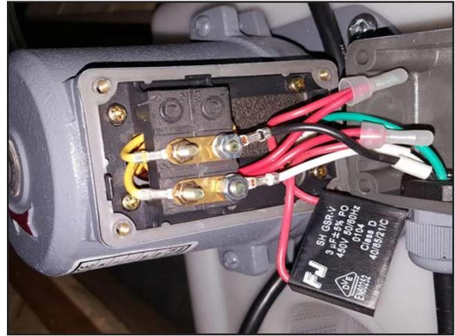
Figure 50. Pump motor wiring and capacitor (M2).
