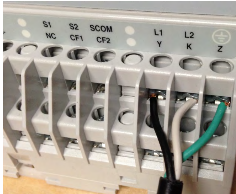
Figure 1 - Temporary Power Connection
